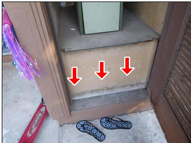
2.1 Item 1(Picture) Moisture stain
