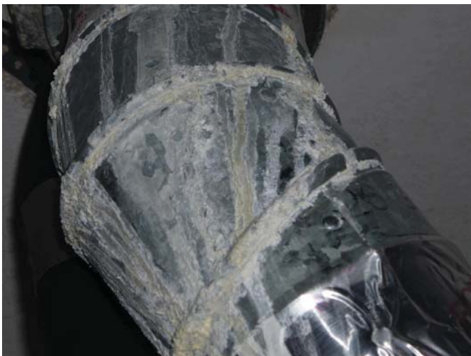
Corrosion heater vent.
