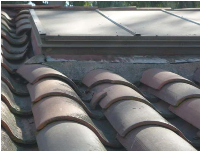
Cracked mud at skylight, cracked tiles.
