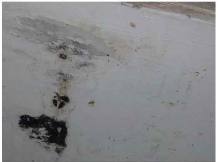
Probable mold growth HVAC platform.
