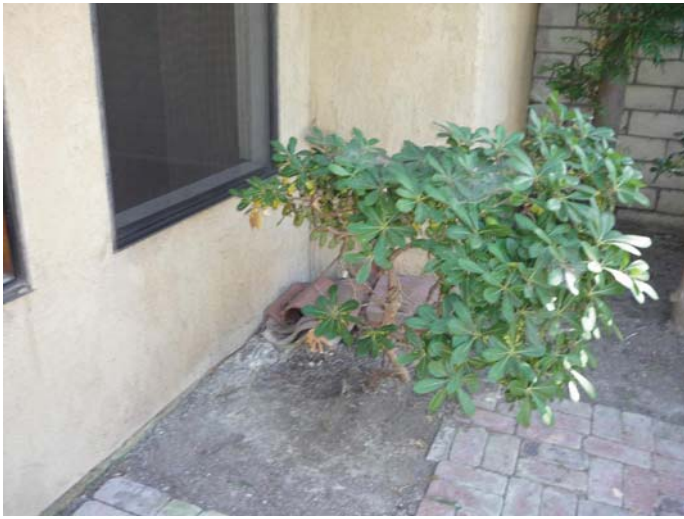
Soil too high at rear yard.
