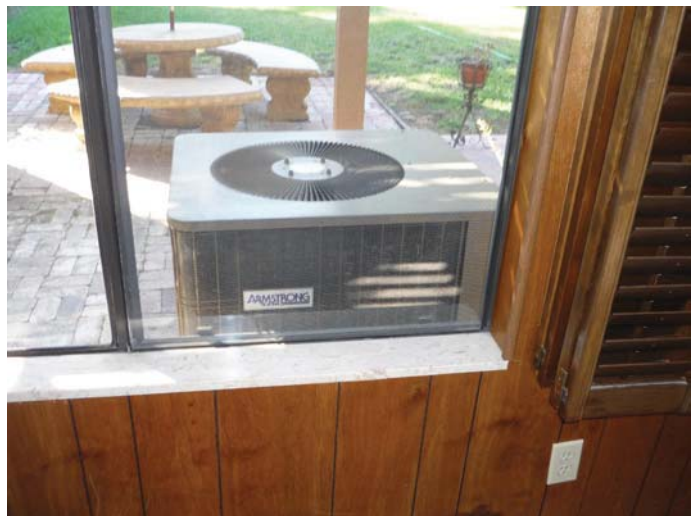
Poor AC location.
