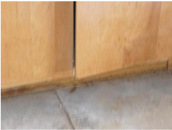
Moisture stains at garage cabinet base.
