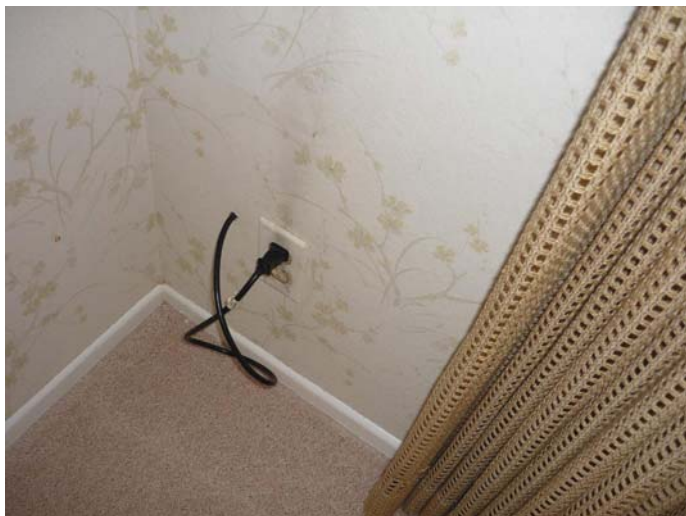
Improper wiring dining.
