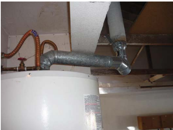
Vent negative slope and touching combustible.
