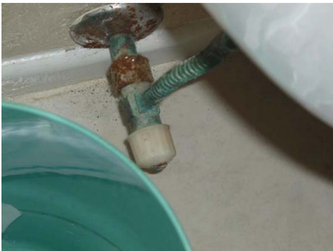
Corrosion at toilet valves.
