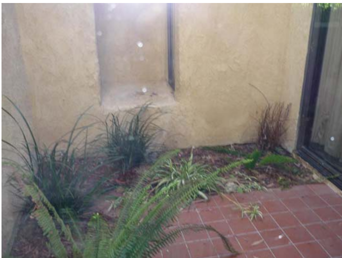
Soil too high to weep screen interior patio, drain not located.
