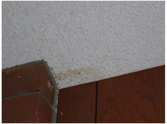
Ceiling stains at fireplace.
