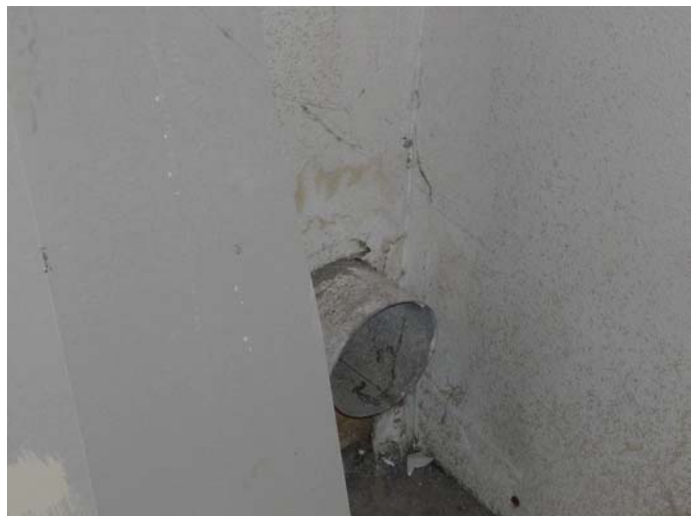
Moisture stains garage wall.
