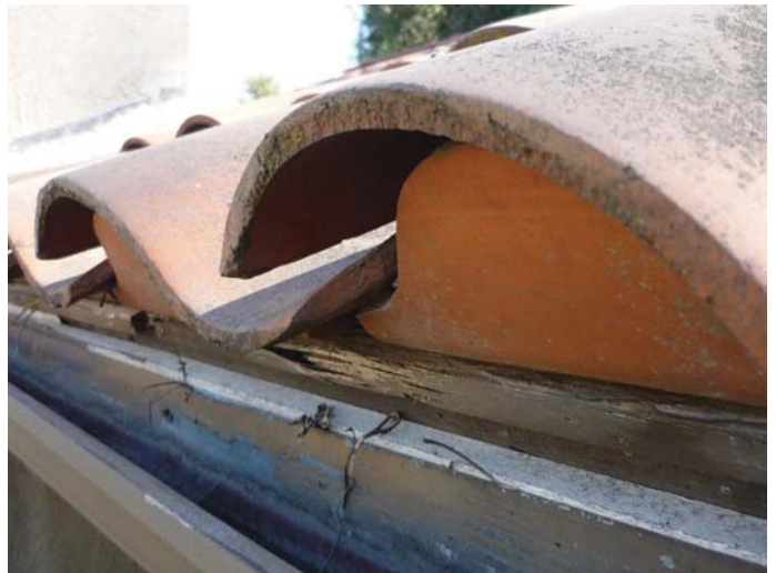
Short paper with missing edge flashing and moisture damage.
