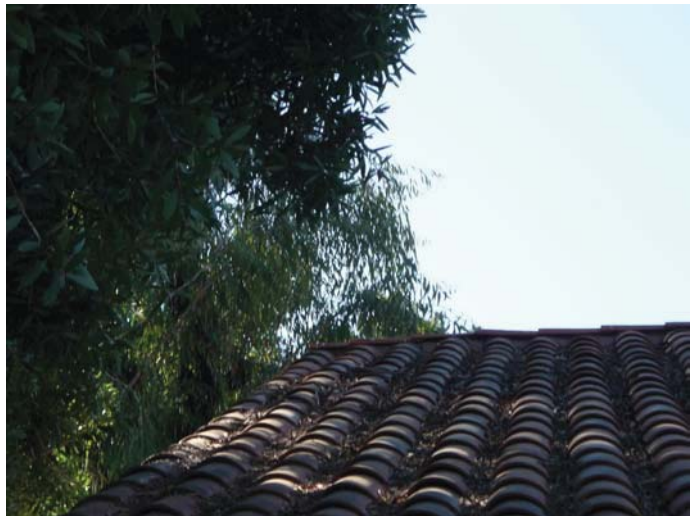
Debris on roof from neighbor trees, trees over roof.
