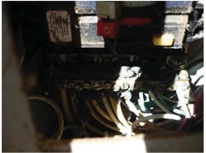
Paste at aluminum wiring at panel.
