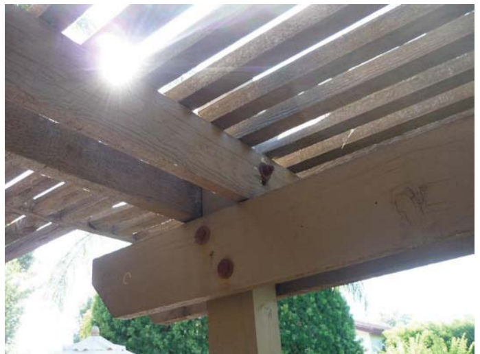
Corrosion at cover fastenings.
