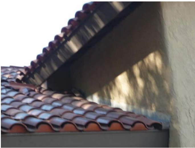
Broken and displaced tiles.
