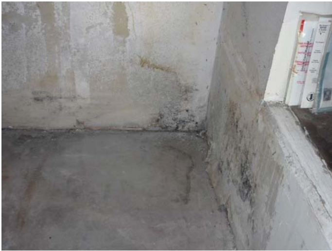
Moisture stains and probable mold growth laundry and water heater area.
