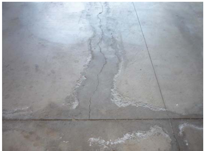
Garage slab crack.
