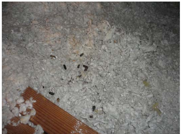
Rodent droppings attic.
