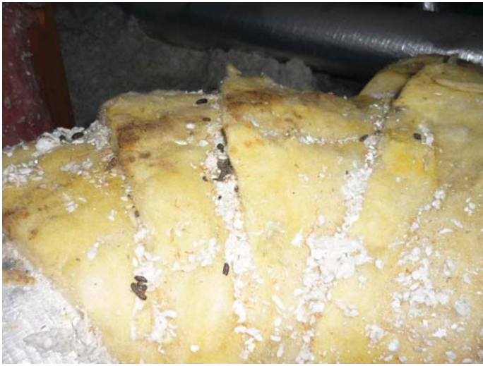
Rodent droppings attic.
